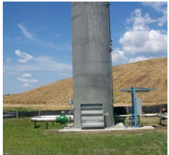
Landfill Gas Recovery Facility - Newark, MD
